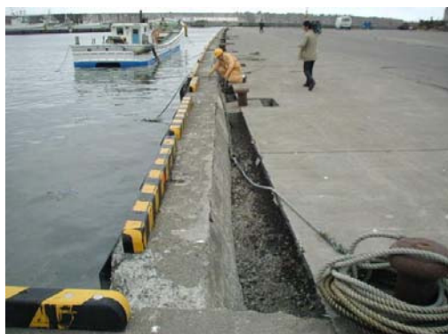
Fig. 2.13 Seaward movement of quaywall during the 203 Tokachi-Oki earthquake
