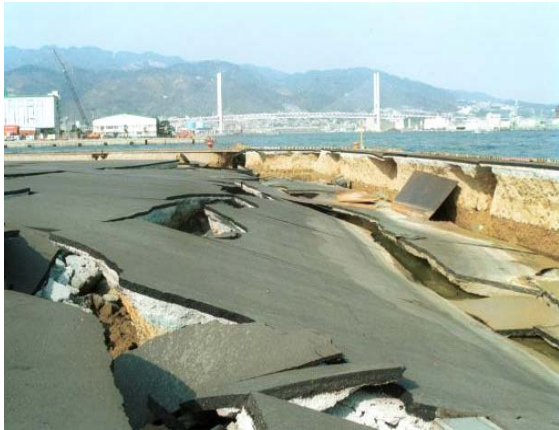
Fig. 2.3 Extremely extensive damage of apron pavements during the 1995 Hyogo-ken Nanbu (Kobe) earthquake
