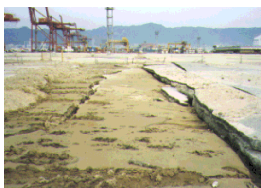
Fig. 2.10 Sand emersion near container cranes [1995 Hyogo-ken Nanbu (Kobe) earthquake, Port Island]
