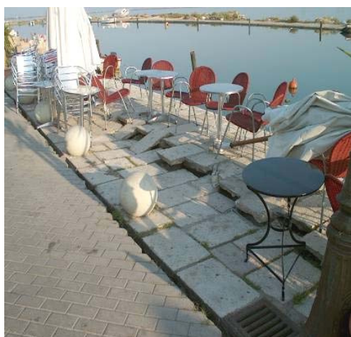
Fig. 2.15 Backfill settlement behind quay wall and damage to apron pavement in the city's port during the 2003 Lefkas earthquake
