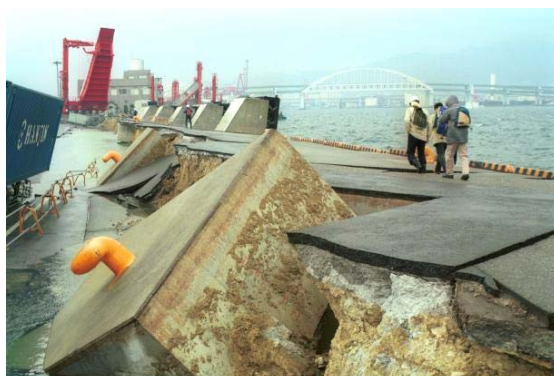
Fig. 2.14 Turnover and extensive tilting of quay-walls during the 1995 Hyogo-ken Nanbu (Kobe) earthquake
