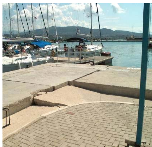
Fig. 2.16 Backfill settlement (25cm), seaward sliding and tilting of quay walls in the city's Marina during the 2003 Lefkas earthquake
