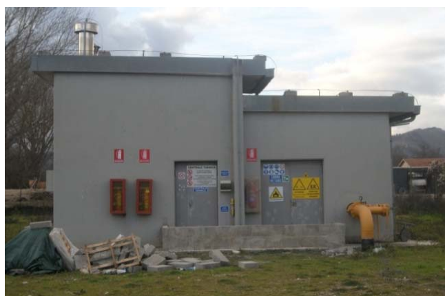
Figure 2. M/R Metering/Pressure reduction station in Onna (L'Aquila, Italy)
