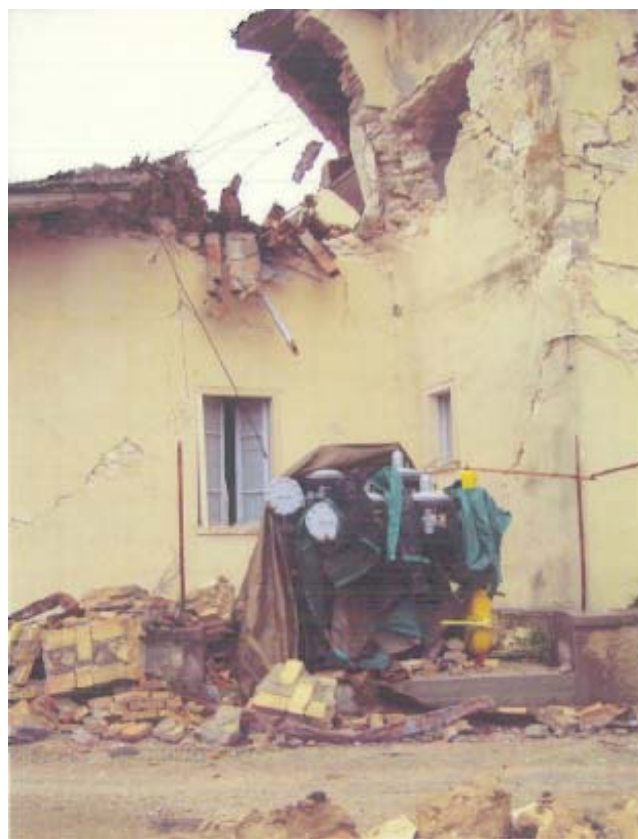
Figure 3. GR housed in a masonry kiosk closed to building and damaged following the 6 th April 2009 earthquake.
